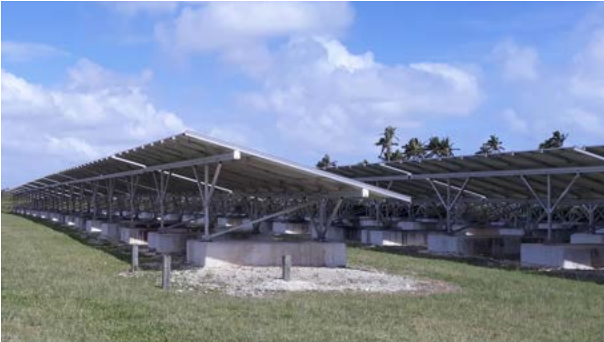
Concrete foundations of a solar farm in Tonga, designed to withstand Cyclone winds.
