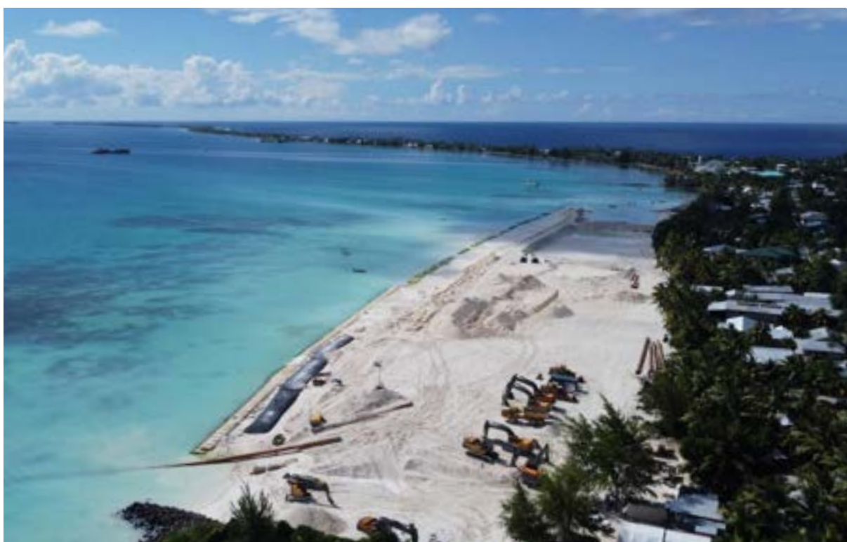
Land reclamation on the lagoon foreshore of Funafuti Atoll in 2023 to create elevated land designed for 2100 sea-level rise scenarios, part of the Tuvalu Coastal Adaptation Project (Source: James Lewis, Intercoastal Consulting).
