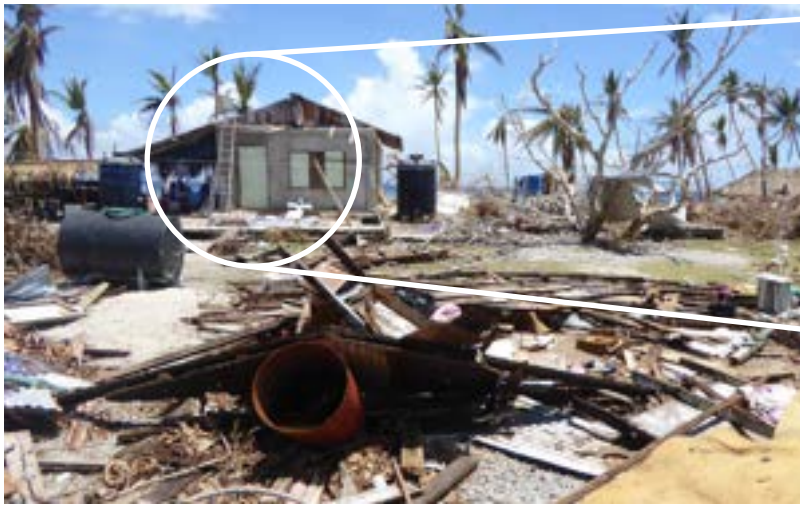
Homes destroyed by Typhoon Maysak in the Federated States of Micronesia. Note: people sheltering in the relatively resilient concrete structure in the background.
